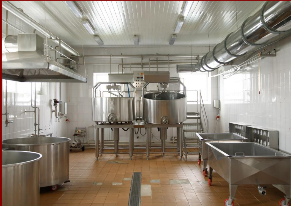
Partition and Ceiling – PUF Panels
