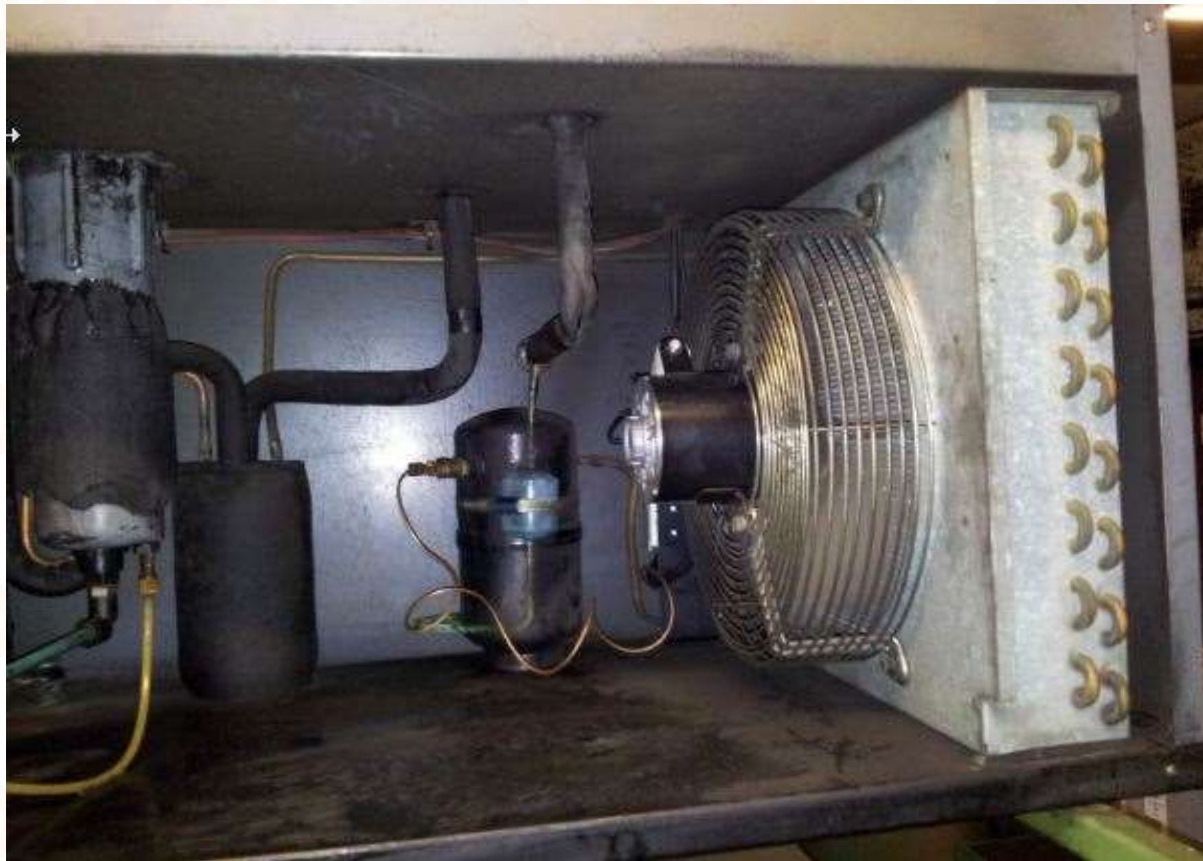
Inside picture of Refrigerant air dryer
